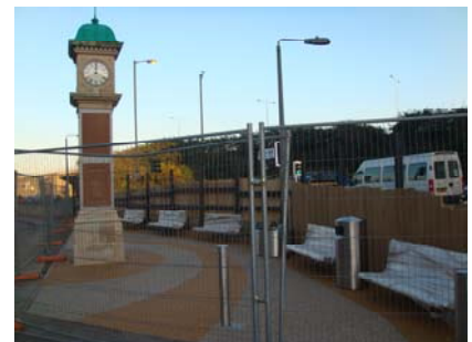
Work on the Sunbury Clock Tower at Sunbury Cross is nearing completion.
